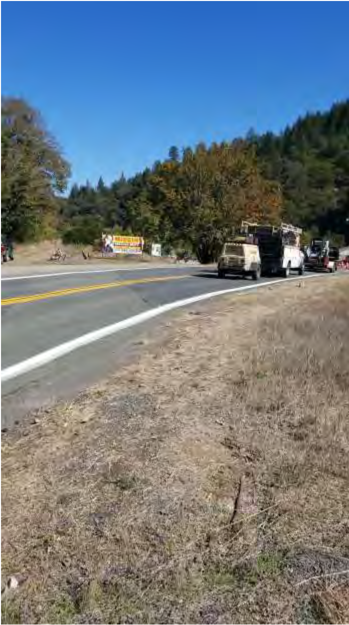
MP 152.2 Covelo road crossing completely removed.
