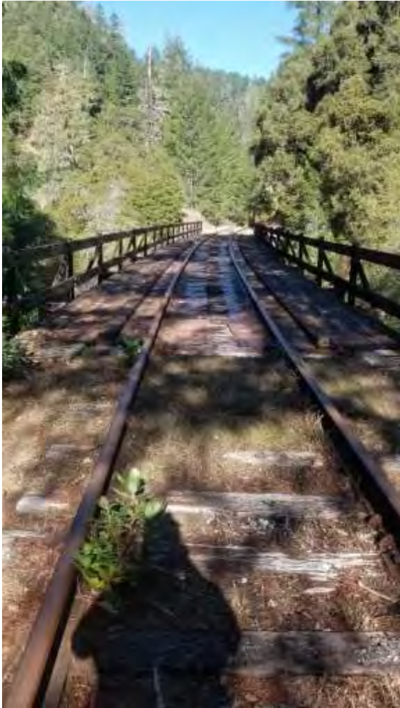
Bridge 147.1 deck ties good condition rail 131 lb and good condition the Metal girder is in good condition, concrete posts are in good condition
