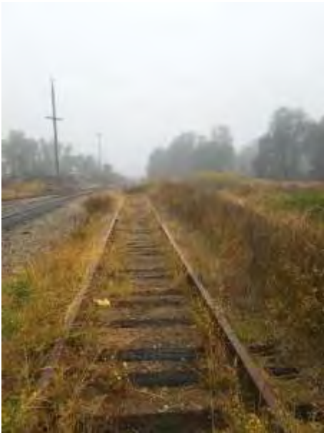
Milepost 139.8 still in Willits yard Vegetation: Poor Ties: Good Rail:132lb. Good Condition
