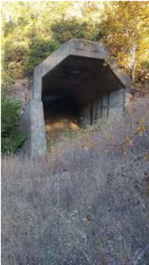
Collapsed tunnel, milepost 145.9 tunnel approximately 400 ft long
