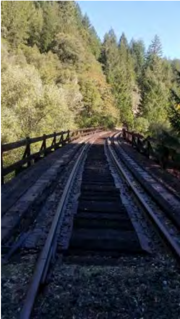
Bridge milepost 147.8 160 ft long, 131 lb rail in good condition. Deck ties are in good condition, metal girders are in good condition concrete pilings are in good condition.
