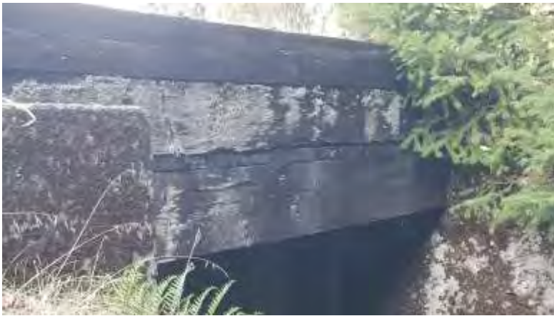
145.1 bridge 20 ft long concrete post in good condition, timbers, and cap in good condition
