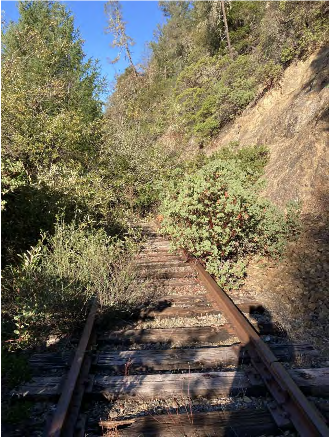
Milepost 150.3, 110 lb rail in good condition. The tie condition is good but would need joint ties for class 1
