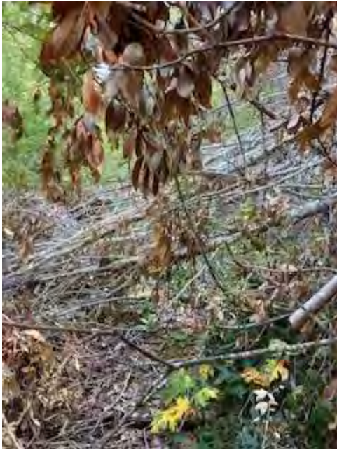
Milepost 149.1, vegetation condition extremely poor. 110 lb rail in good condition, tie condition covered.
