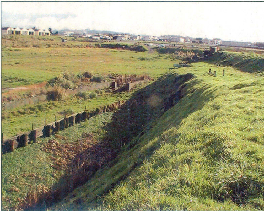
View of the oversteepened slope of the northern dam wall above Pond 7
