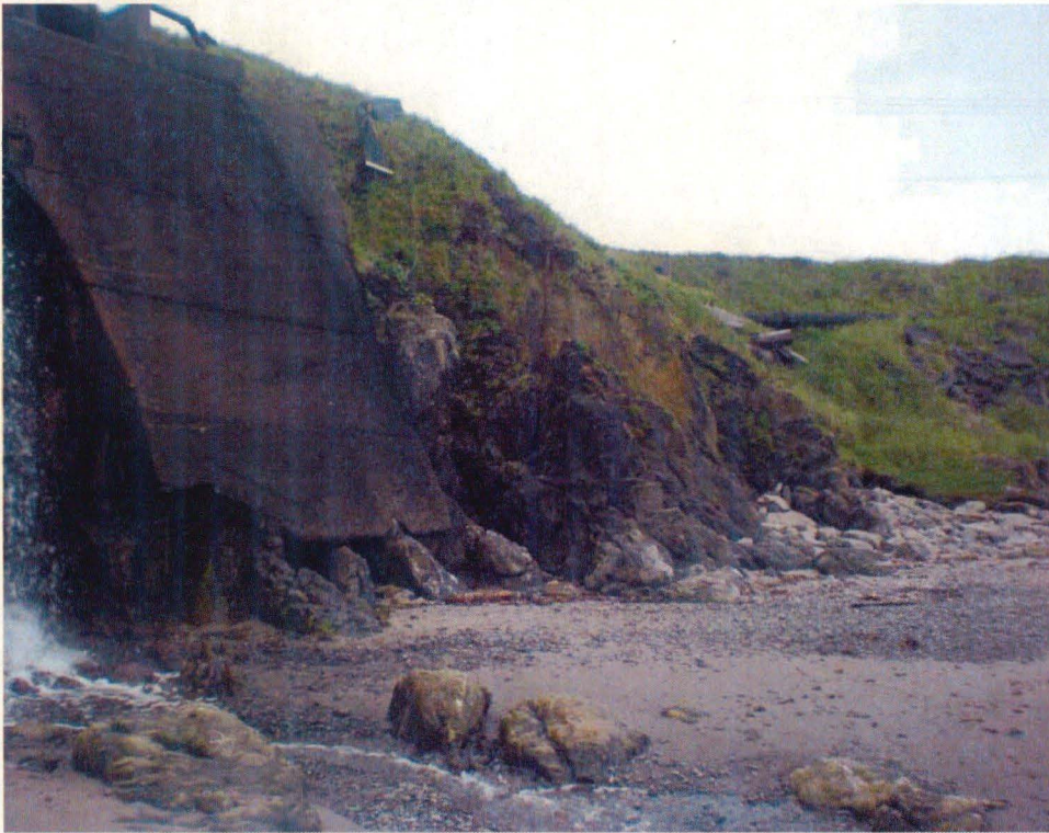
View of the western wall including the spillway and the cribwall showing beach erosion and shoreline loss
