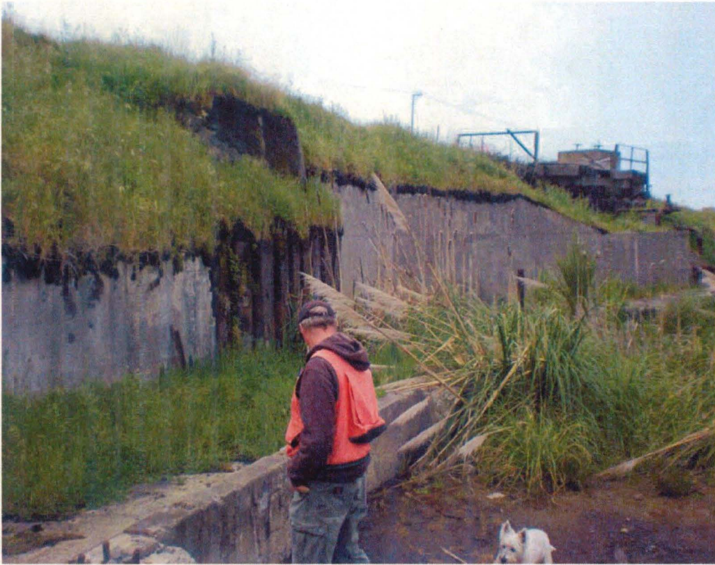
Eroding concrete retaining wall along the north wall showing extensive leakage
