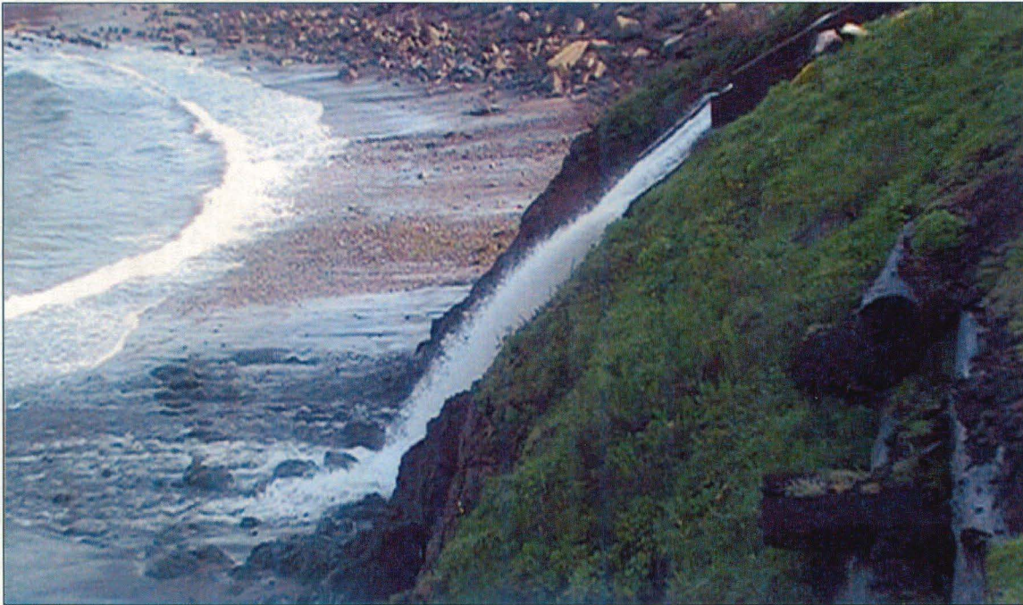
View of the cribwall and the spillway discharging directly on the beach
