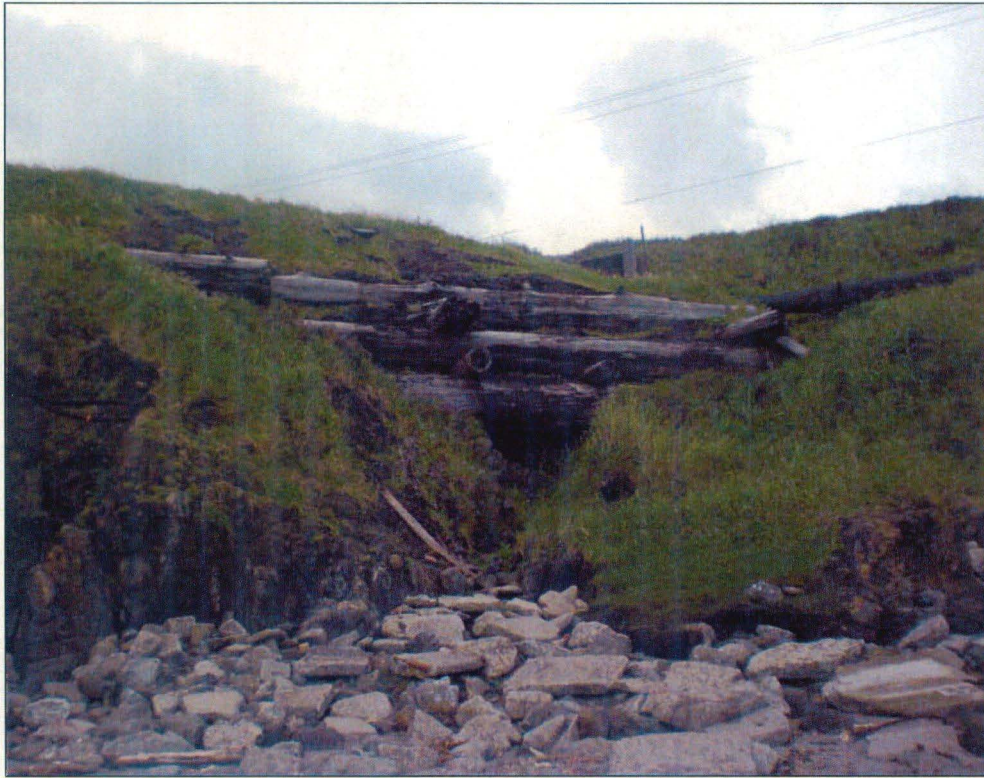
Crib wall on the western dam wall exhibiting soil loss and cavity developing amongst the cribs
