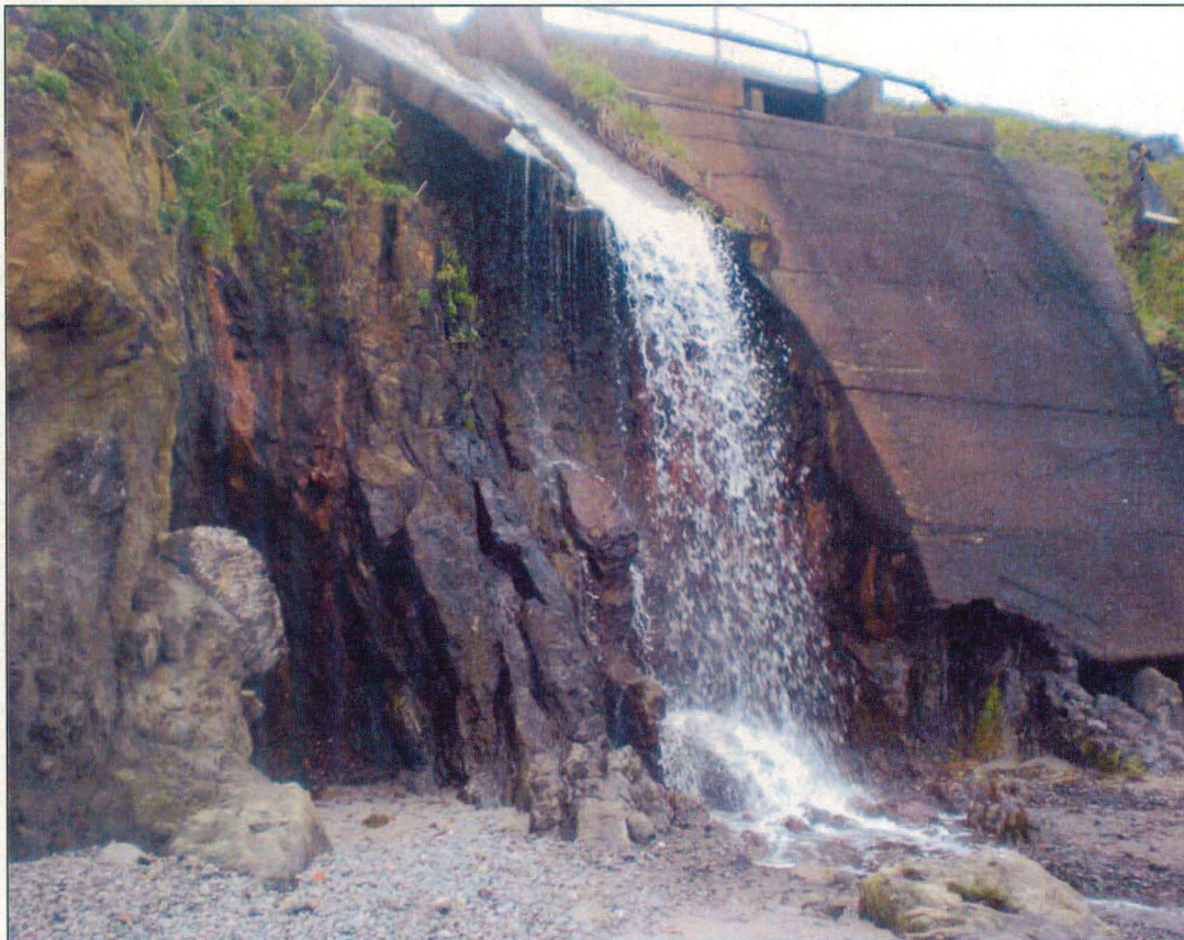
Spillway showing beach erosion and damage to the spillway concrete flow structure
